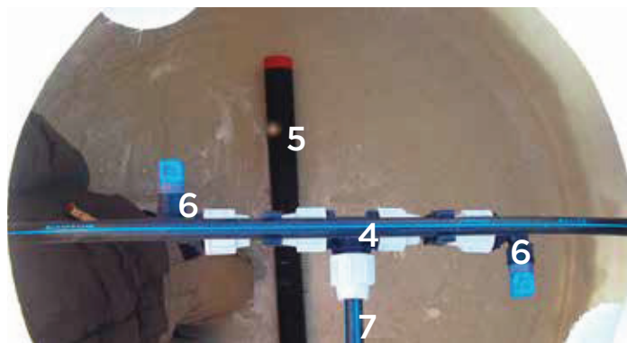
Spredesystemet i biofilteret
